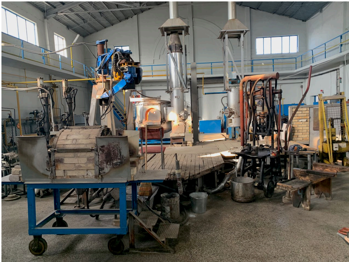
Figure 3 Equipment and energy consumers
