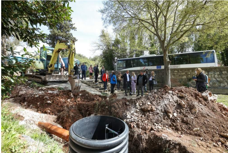
Rain gardens and a smart drainage system installed in the garden of a school in Zadar
