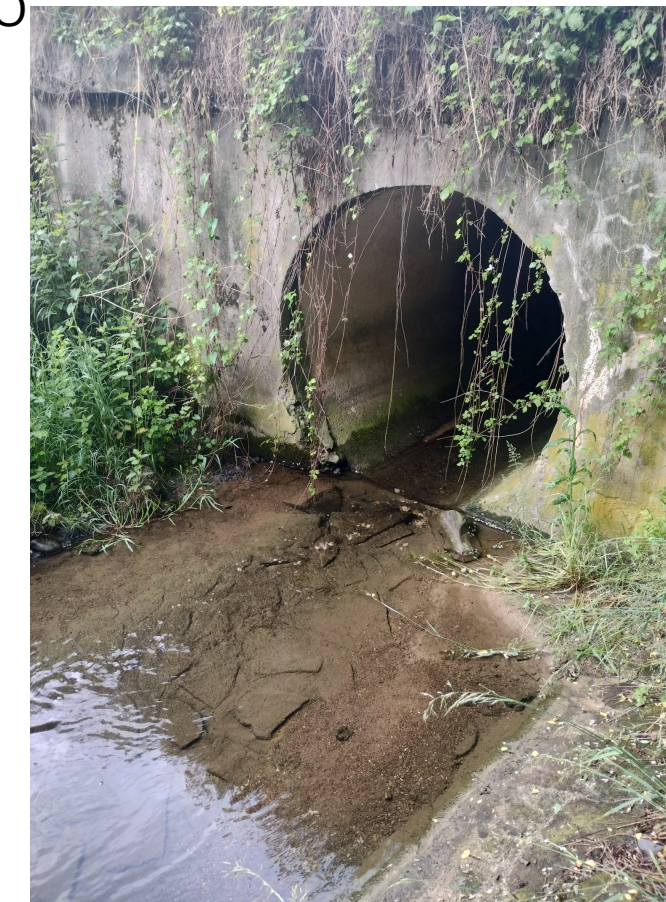
Outlet of surface runoff from the Military Airport Sliac, SK
