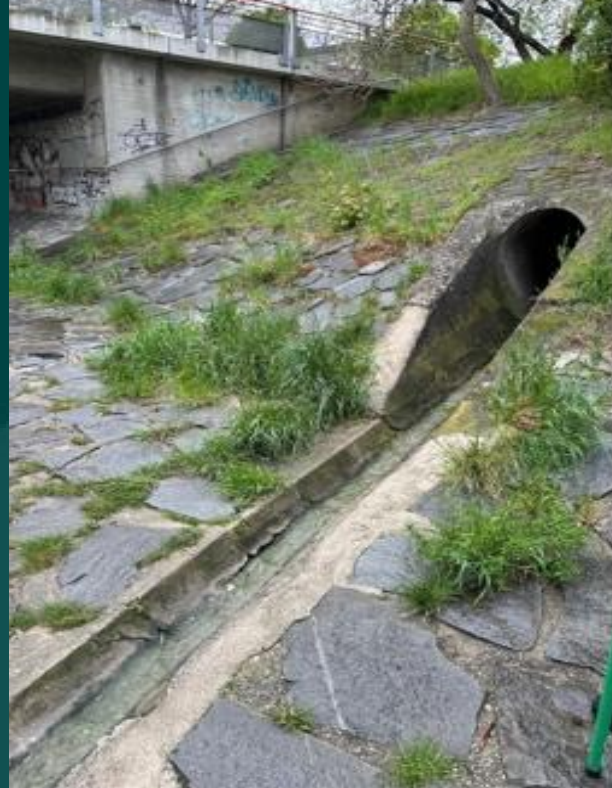
Urban storm runoff water, Liesingbach, AT
